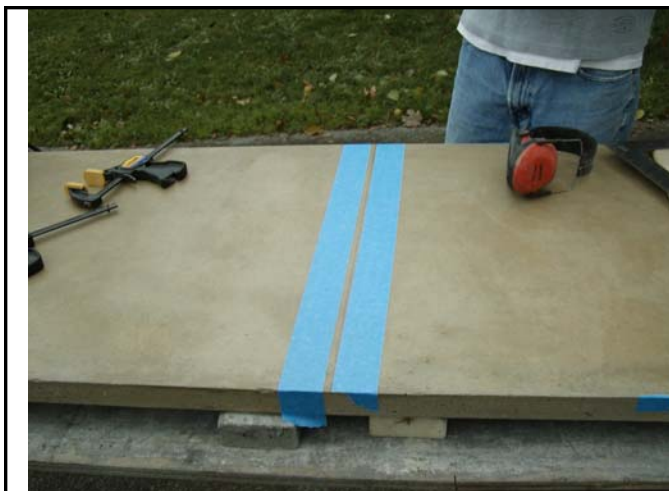
Masking tape is used to protect the slab from the pad of the saw as this piece is being cut. However, masking tape can also pull up some of the shop-applied sealer and should be repaired and resealed before the counters are used.
