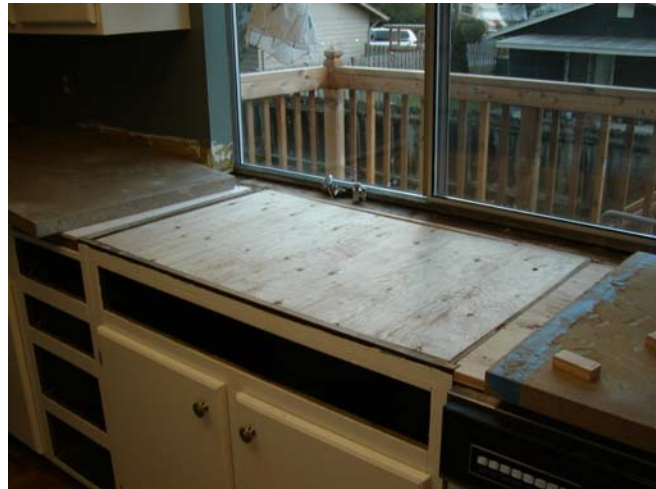
A plywood substrate is used over the dishwasher and the sink cabinet. Note that the substrate is inset flush with the tops of the cabinets, to avoid an reveal formed by the plywood sitting on top of the cabinets. The plywood is supported underneath by corbel-type bracing.
